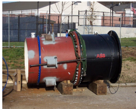
60-inch magnetic flowmeter being installed in Philadelphia, PA
