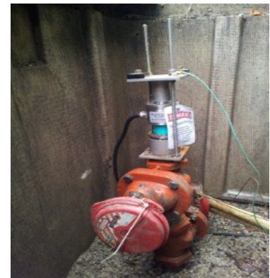
Insertion magnetic flowmeter in use on a 30-in. pipeline in Birmingham, Al
